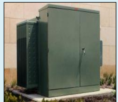
Figure 2: Above is an example of a pad mount transformer. This would not trigger referral to us.
