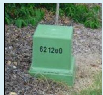
Figure 3: Above is an example of a service pillar. This would not trigger referral to us.
