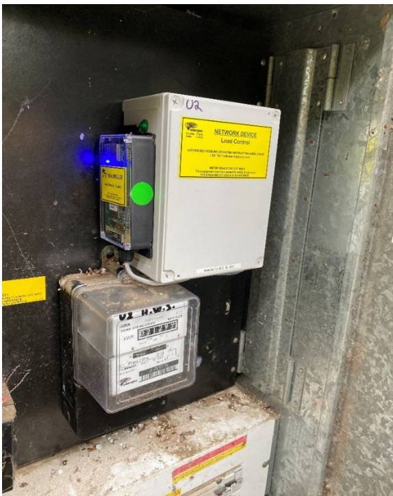
Image 1: Load control relay and comms device in-situ
