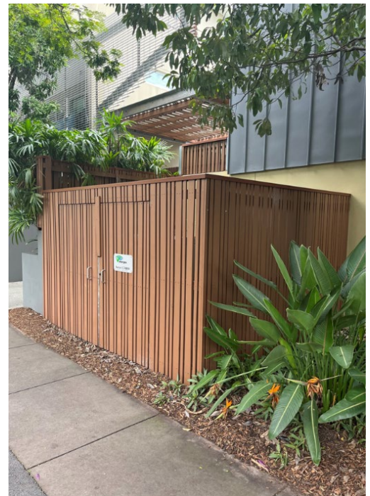
Figure 2. Example of creating more visually attractive Padmount Transformer.
